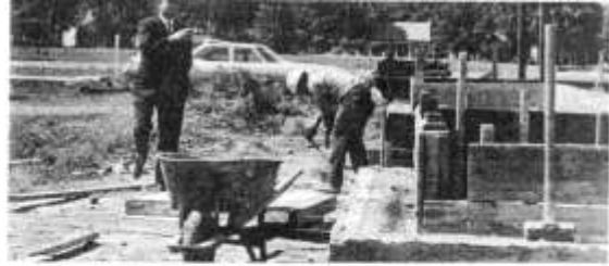
Mr. Draut takes a moment from his busy schedule to watch the workers constructing Waggener's new gym.
